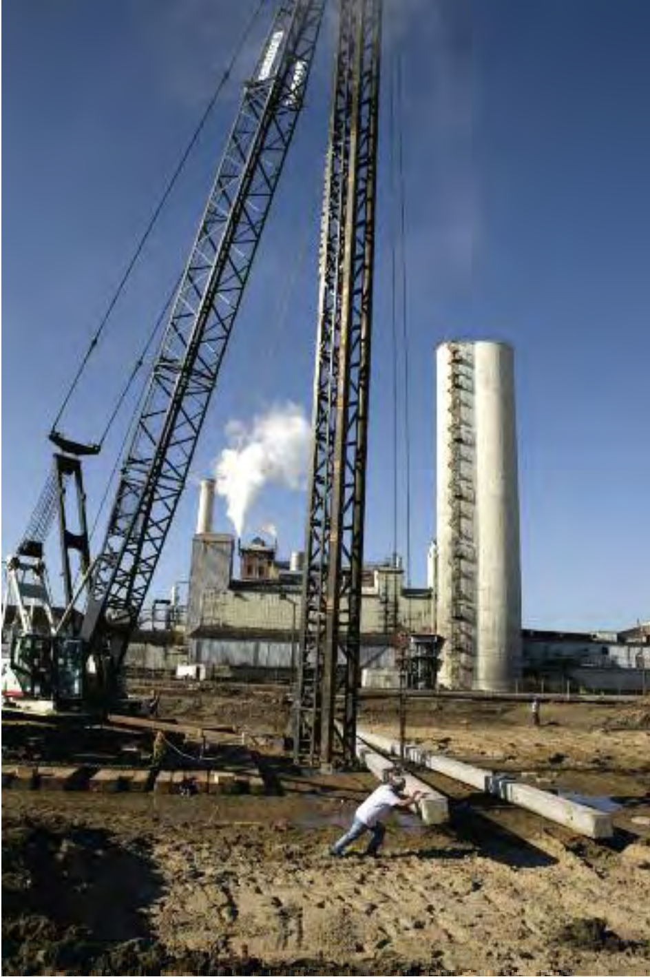
Construction progresses on the new Louisiana Sugar Refining plant in Gramercy, La., next door to the Imperial Sugar plant. The new plant is a joint venture of Louisiana Sugar Growers, Cargill and Imperial Sugar.
