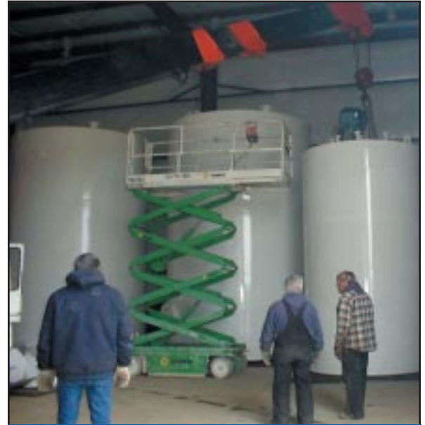
Fuel tanks are installed at the new Clinton County Bio Energy plant, which should be operational in May 2006.
