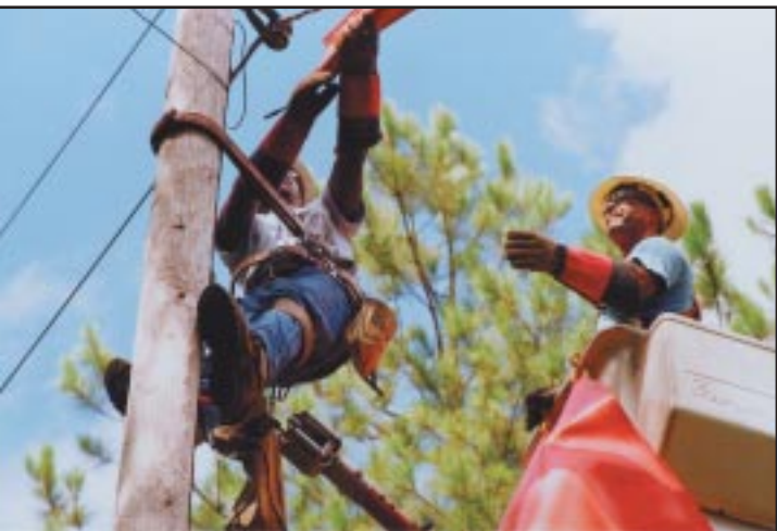
Skilled linemen keep Walton's infrastructure in good shape while holding down service costs for co-op members.
